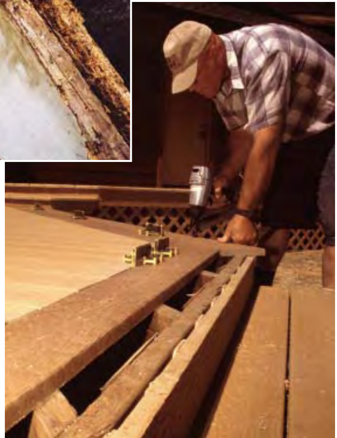
Figure 2. On this deck, water got between the fascia and rim, partially rotting the fascia and completely destroying the rim (above left). When the fascia was removed, the rim collapsed. Here (above), on a pressure-treated frame, the author installs composite decking that will completely cover the fascia and rim, avoiding this potential collection zone. The lattice separating the fascia and rim joist will also help to drain away water.
