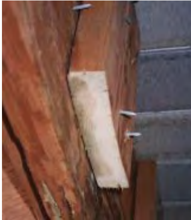
Figure 1. Pressure-treated hem-fir lumber is incised to increase penetration, but often the colored preservative barely soaks in at all, as is evident on this piece of blocking. The end cut should have been coated with preservative; the brown staining visible on the end grain is a sign of rot.
