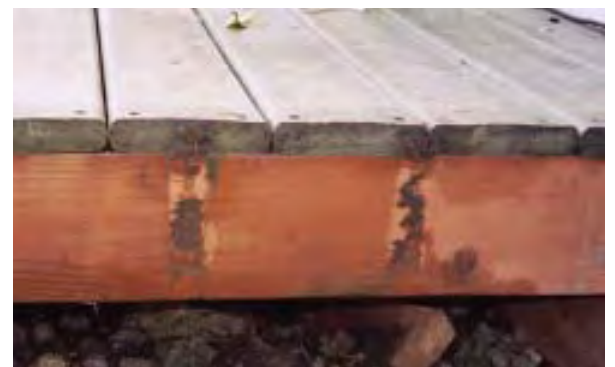
Figure 7. Nailing balusters to the rim joist creates pockets that trap moisture and debris, which can cause rot.
