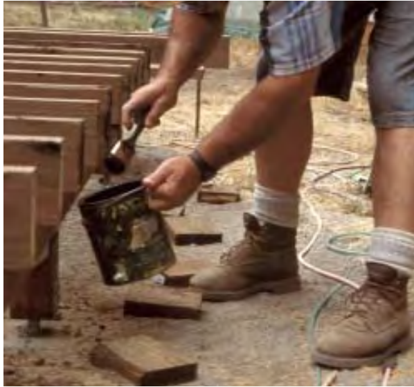
Figure 8. It's a good idea to coat pressure-treated yellow pine end cuts with extra preservative. With hem-fir, which doesn't accept pressure treatment well, it's an absolute necessity to do so.
